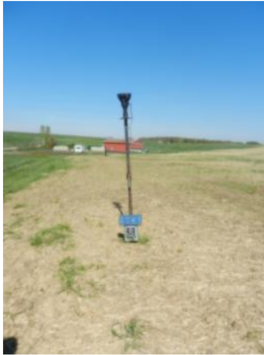
Gas flare solar powered device at Landfill 1
