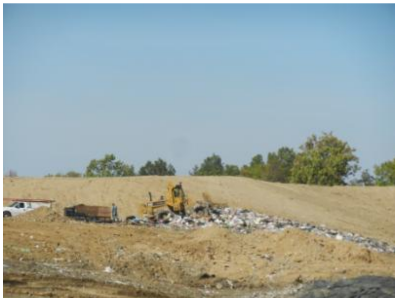
Landfill pile being crushed and shifted. Landfill is almost at maximum height prior to cap off
